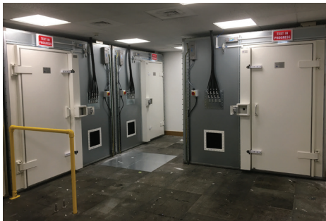
NTD Shielding Services application of custom-designed RFI shielded chambers. Each houses a comprehensive electrical wiring system with incoming power lines located behind a pneumatic door as pictured here.
